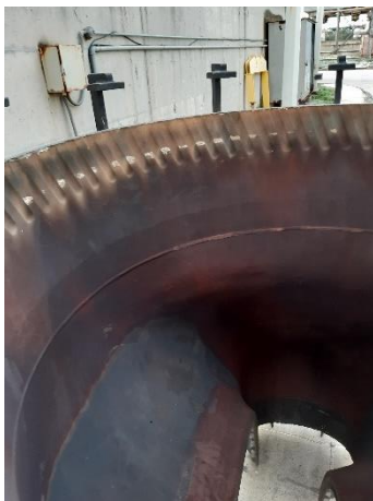
Typical TBC chipped off the contact with Inner Liner
