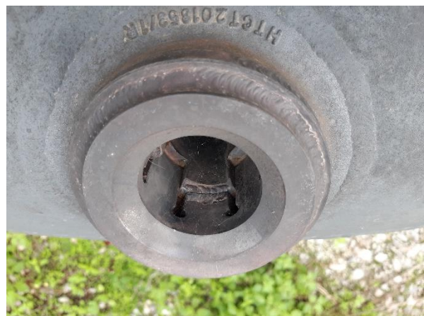
Flow dividers bushes Overview – Typical operation weld cracks
