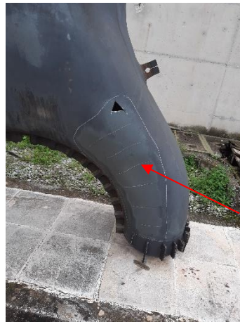
Huge Deformation main body Compressor Side
