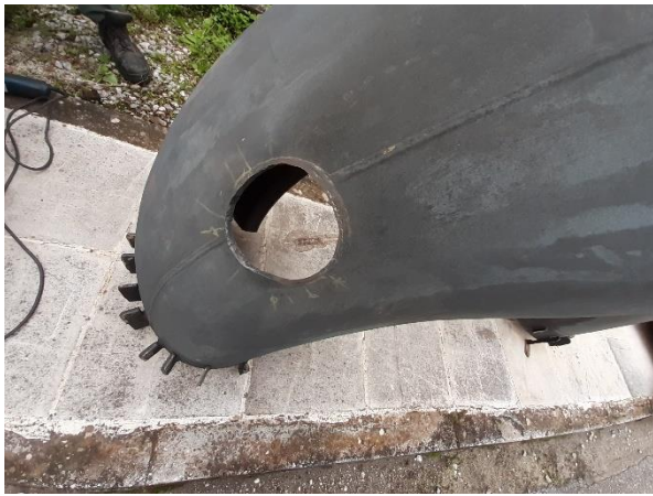
Inspection Hole -Typical fretting
