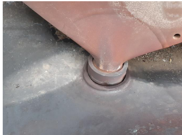
Flow dividers bushes Overview (internal hard face coating expected)
