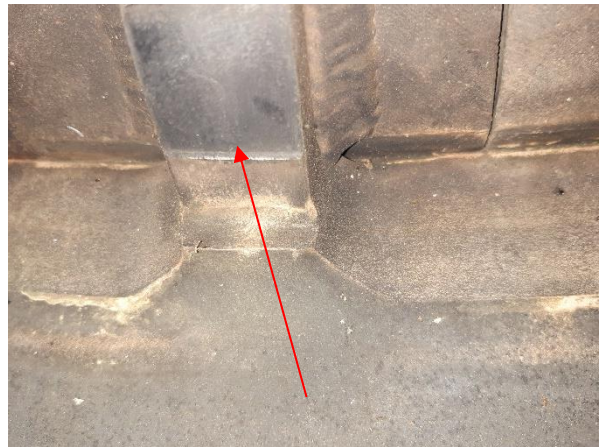
Compressor Suspension Ring – fretting contact surface (2-3mm)
